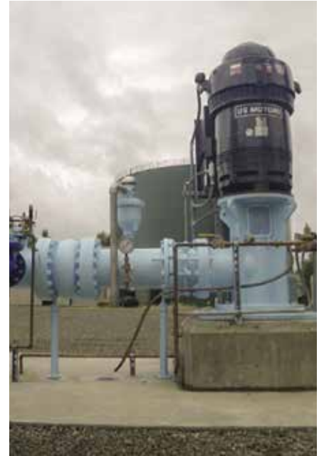
Rockwood Water PUD Groundwater System
